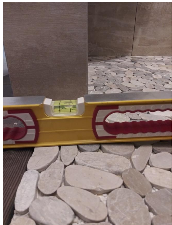
Water landing at this shower entrance will flow out into the room (left), not back into the shower (right).
